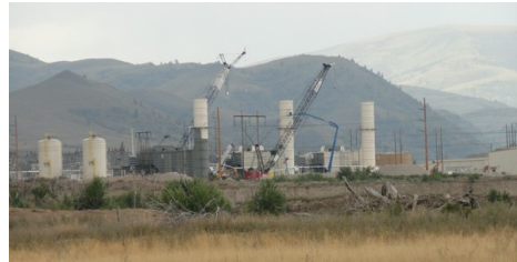
Dave Gates Generating Station | Corval Group
